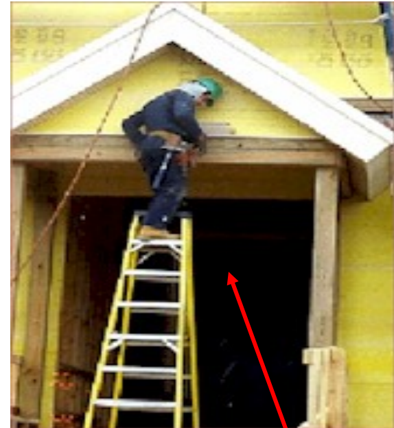
Improper use of the top rung of a step ladder
