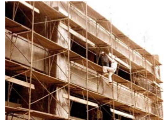
Do not access by cross braces
