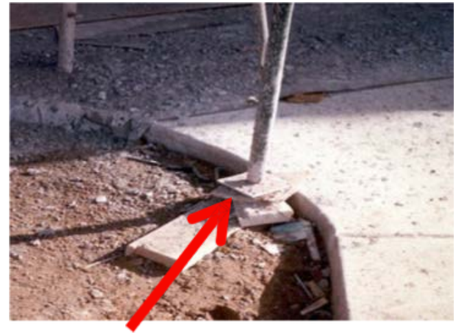
This support is not adequate!
