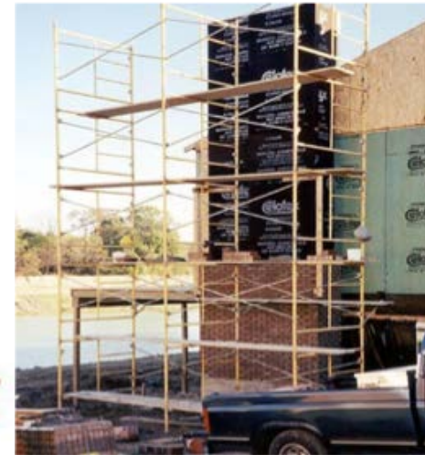
This is not a properly constructed scaffold!
