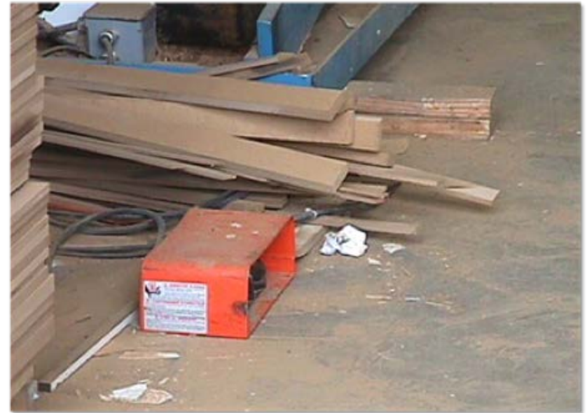
Poor housekeeping can cause trips.
