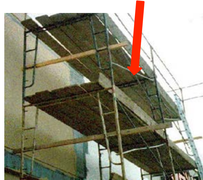
Large gaps in front edge of platform
