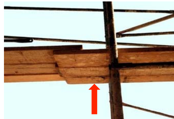
Planks not properly overlapped
