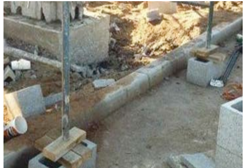
Inadequate support? In danger of collapse
