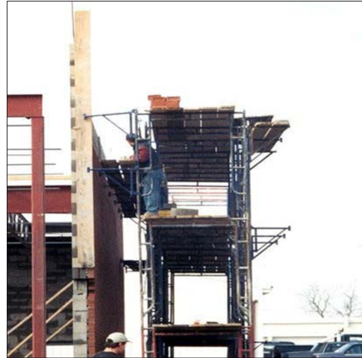
The ends of this scaffold are not properly guarded.
