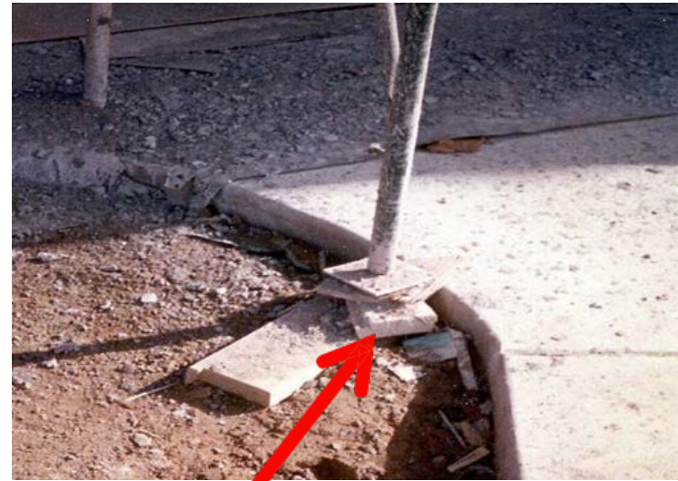
This support is not adequate!
