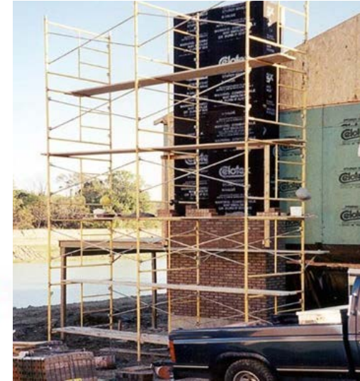
This is not a properly constructed scaffold!
